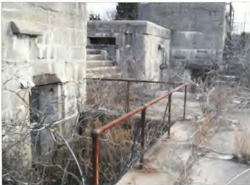
Figure 5.26. Existing historic safety railing at Battery Urmston is fabricated of pipe rail sections and ball joint connectors. After treating corrosion and restoring the historic finish, infill panels should be installed where there is a vertical change equal to or greater than thirty inches in order to provide greater safety at the large openings below the top rails (Olmsted Center, January 2009).
